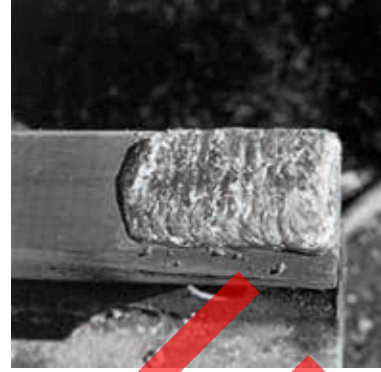
Figure 5 – BUILD-UP - Worn Rail End Rebuilt Past Original Dimensions-It Will Be Ground Prior To Service.
