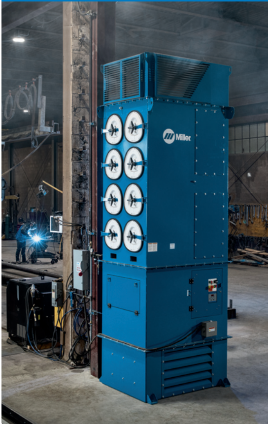
Before: Lingering weld fume haze
