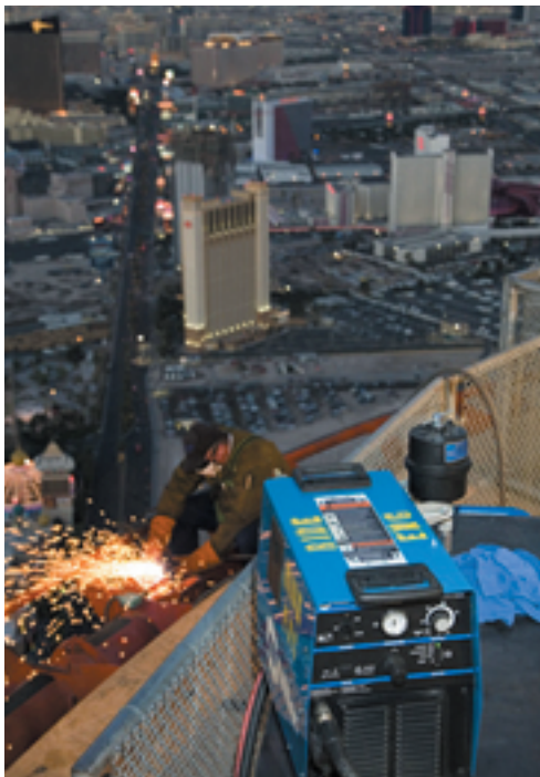
Stratosphere Hotel and Casino ride engineers reduced cutting time by about 55 percent with the Spectrum® 1000 plasma cutter.
